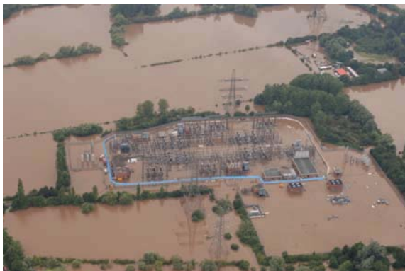
Walham sub-station surrounded by floods
