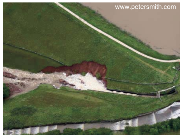
Damage to the masonry channel and dam
